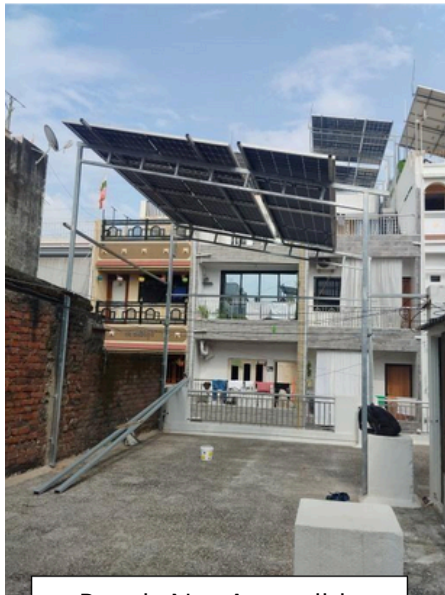
Panels Not Accessible
